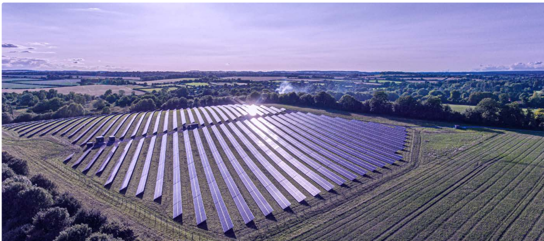
Octopus-managed solar plant in Hampshire, generating 4.5GWh/annum.
